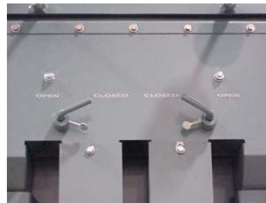
Feed gate valves in closed position
