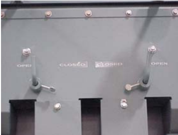
Feed gate valves in open position
