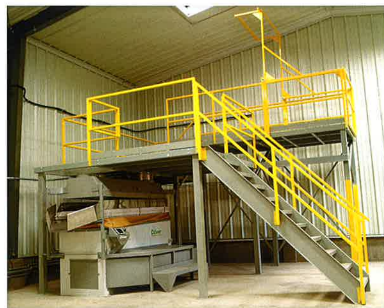
Oliver DVX 307 installed with custom-built catwalk
